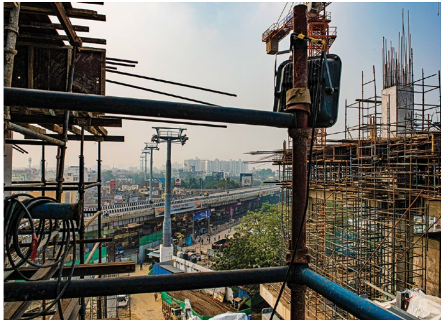
The construction site of Vishwa Samudra Group’s urban ropeway project in Varanasi that spans 3.85 km, with a passenger capacity of 96,000 per day
